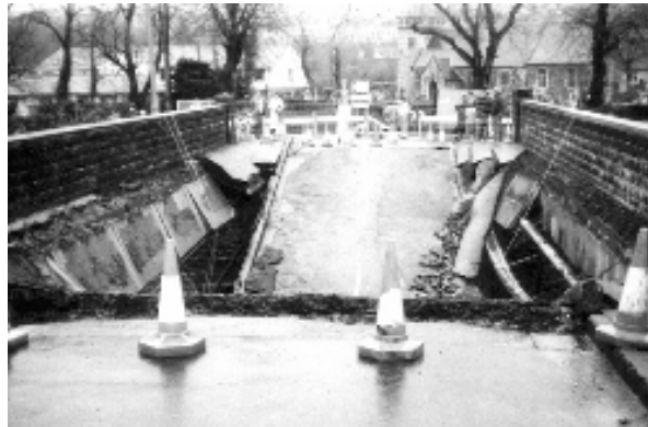
Figure 2.10 Ynys-Y-Gwas at Failure, 1985 15
