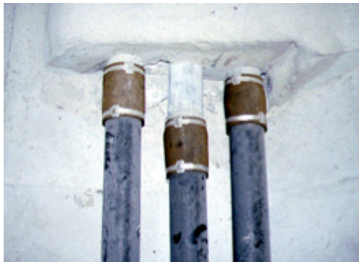
Figure 2.11 Tendon Slip at Deviation Block 19
