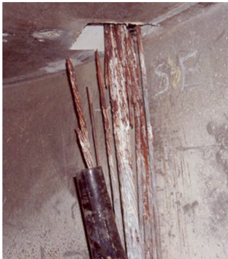
Figure 2.13 Corrosion of Vertical External Tendon 19
