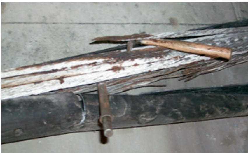
Figure 2.12 Corrosion in the Free Length 19
